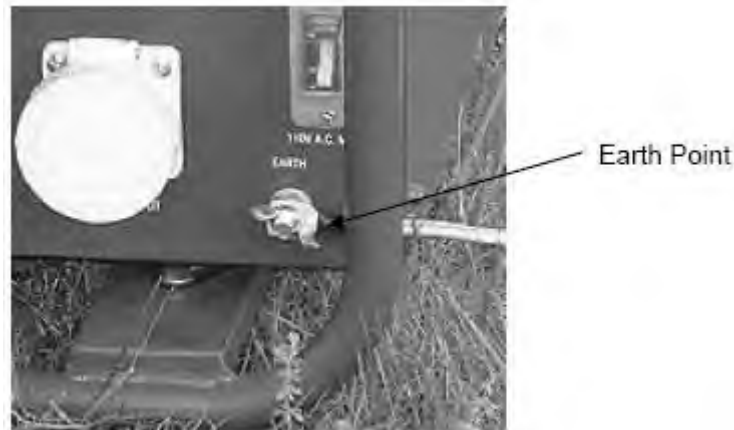
Fig 9 Earth lead connection point
