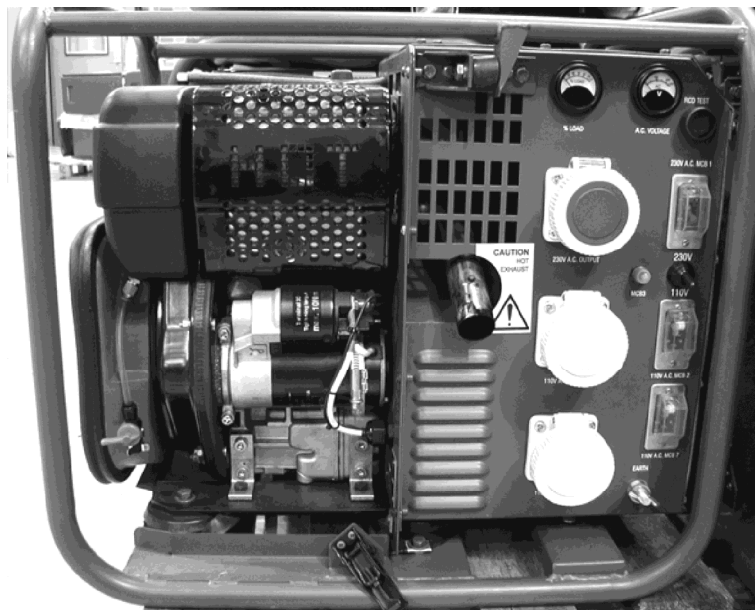
Fig 2 Component locations - AC panel side (acoustic cover removed)
