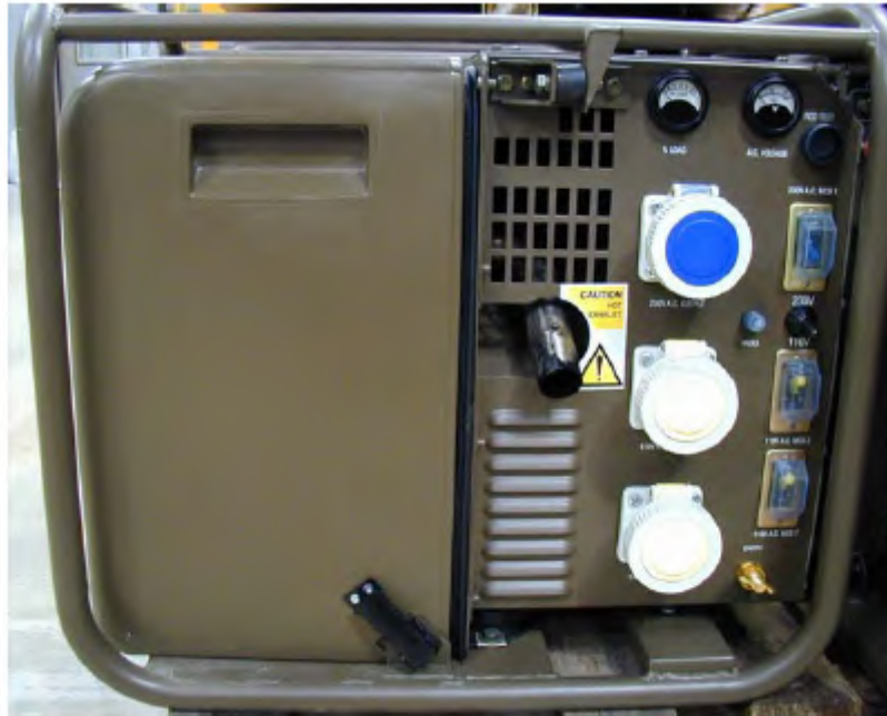
Fig 1 AC panel side (acoustic cover fitted)
